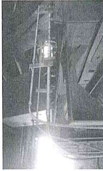
Fixed type DS system for coal Conveyor
