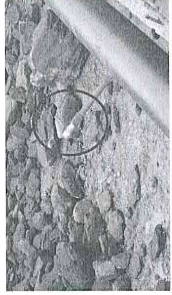
Fixed type DS system at Coal Yard
